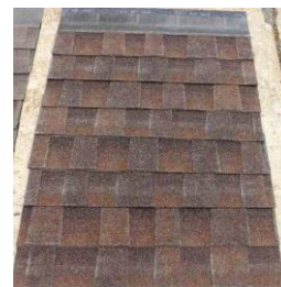
Cutter dust on new shingles
